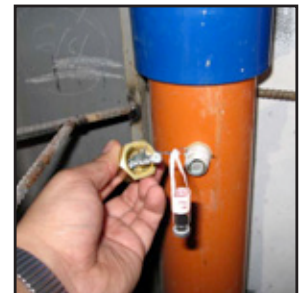
Sampler deployed in a vapor off-gassing pipe
